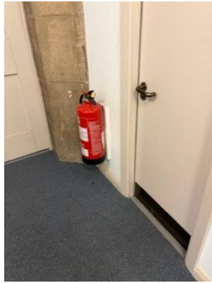
First Floor Lobby – Water TGT 12
