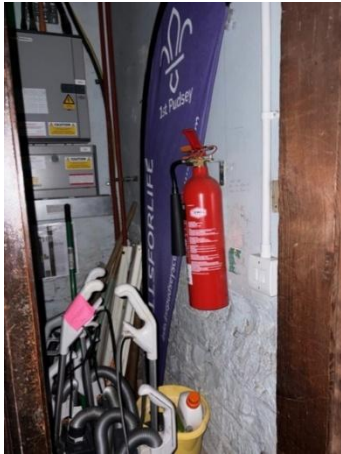
Electrical Cupboard CO2 TGT 9
