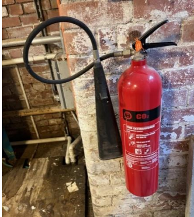
Boiler Room Zone 1 CO2 TGT 15
